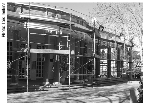
Scaffolding covers the facade of le Petit Trianon as repairs get underway.
